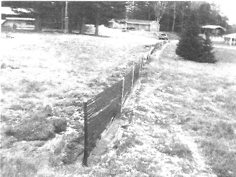
Photo 6: Looking west toward Paquette drive along silt fence. This silt fence is not embedded into the ground (trenched but not backfilled).
