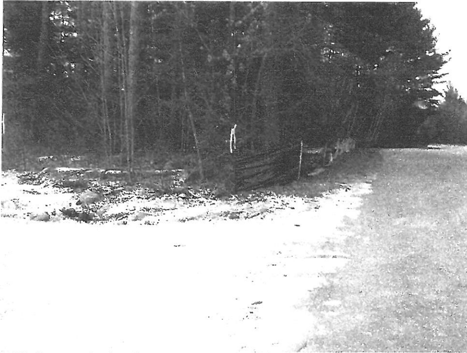
Photo 5: Silt fence south of road entrance on Paquette drive. This silt fence is not embedded into the ground, and appears not to be on the development lot.
