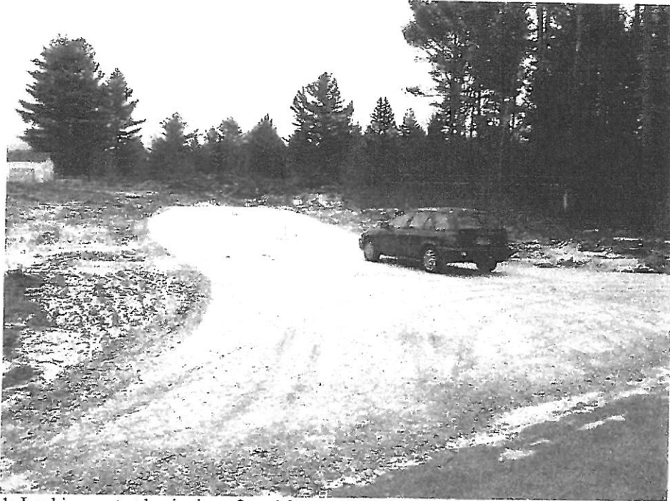
Photo 1: Looking east at beginning of road from Paquette Drive. Crushed gravel has been placed to approximately station 1+45 (145' from the edge of Paquette Drive).
