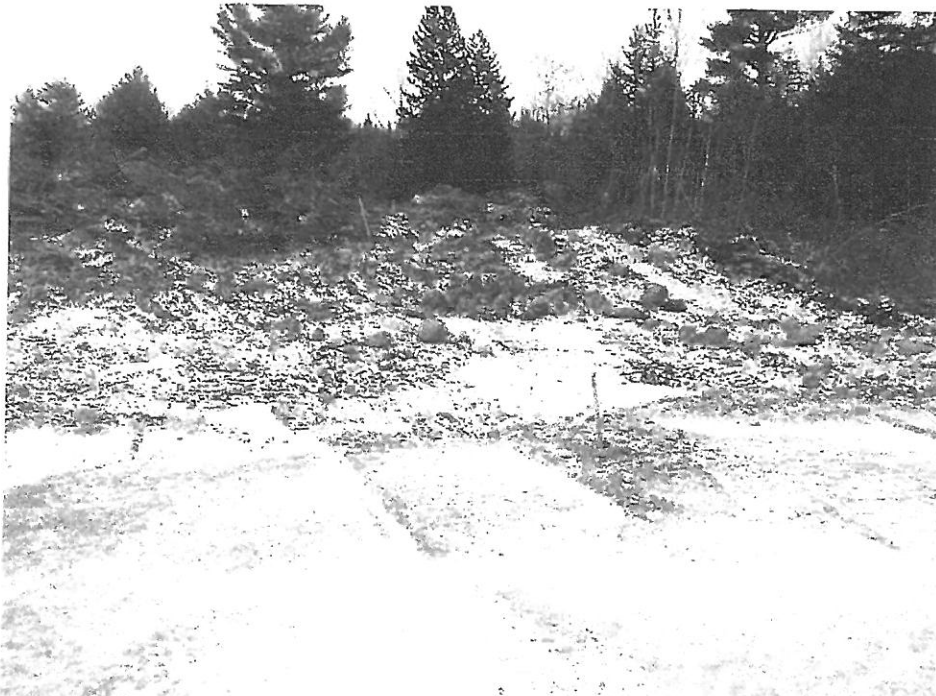
Photo 2: Looking along roadway at end of built roadbed. Bank run gravel has been placed slightly beyond station 1+50 (grade stake in foreground is 1+50).
