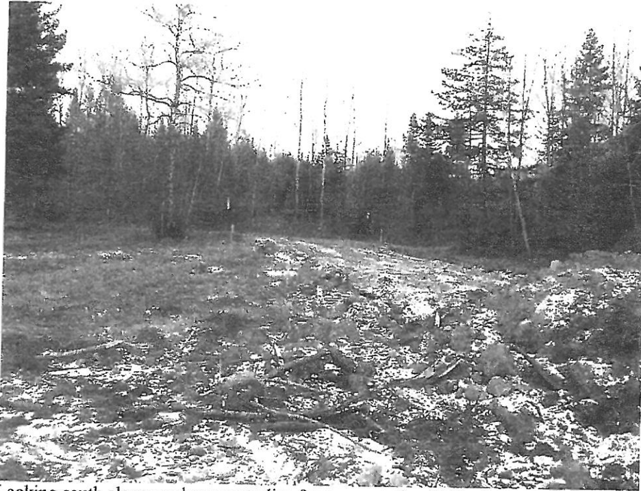
Photo 3: Looking south along roadway centerline from near station 3+00. Some topsoil has been stripped. No work is apparent beyond station 4+50 (at treeline in this photo).
