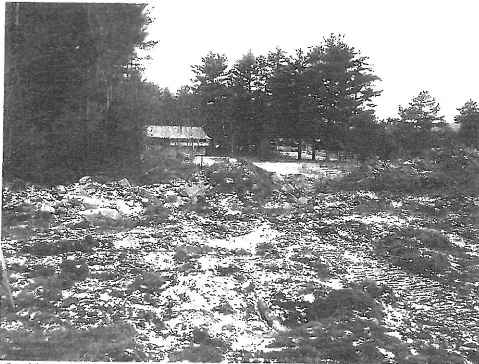
Photo 4: Looking northwest (toward Paquette Drive) from near station 3+00. Concrete debris piled on left and grubbed materials piled on right.
